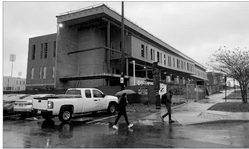
PHOTOGRAPH BY TERESA JOHNSON, COURTESY CAPITAL NEWS SERVICE Construction at Cole Field House at the University of Maryland-College Park on Dec. 9, 2019.
